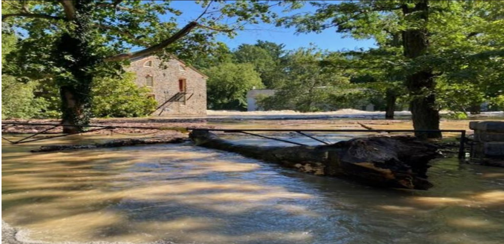
Hurricane Ida (September 2, 2021) high water mark at Howard High School in Wilmington, DE
