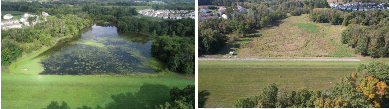
Beaver Creek Dam in East Brandywine Township before (with a 7.2 million gallon pool) and after (operating as dry dam with no permanent pool) the rehabilitation project, completed in 2022.
