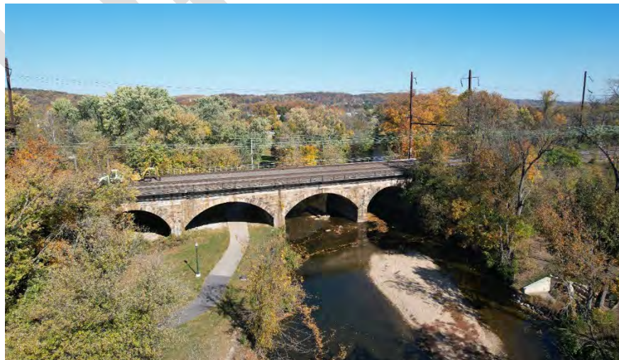
Railroad bridge over the East Branch Brandywine Creek in Downingtown Borough. October 22, 2024. Note the two arch sections are partially restricted due to silt accumulation.
