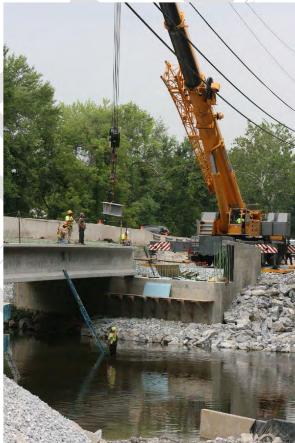
Construction of bridge on US Route 322 over the East Branch Brandywine Creek in East Bradford Township, August 6, 2014. Photo Courtesy of Chester County Planning Commission.
